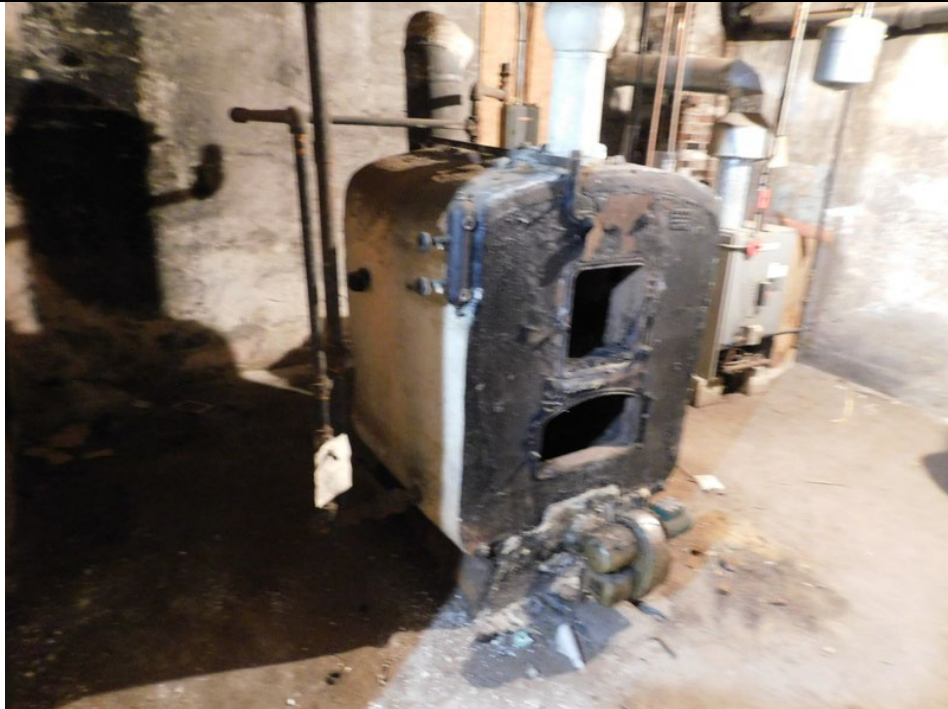
Property overview – TSI on boiler in 518 basement
