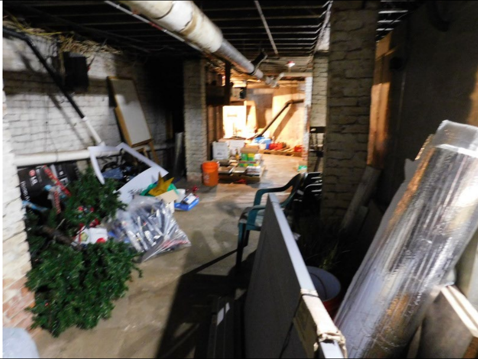
Property overview – TSI along piping in the 518 basement
